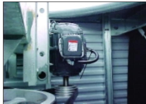
Motor sheave mounted on end of shaft and beyond center point of sheave. Motor shaft eventually snapped.
